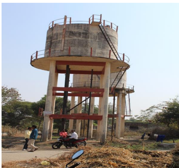
Fig. 3 Elevated Storage Reservoir
