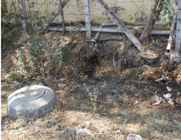
Fig. 8 water logged area
