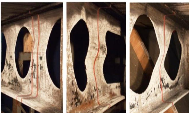
Fig 2. Shear Buckling of a Web Post
