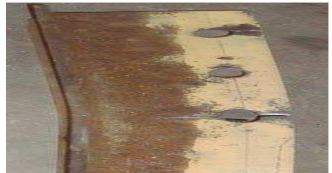
Fig. 4.2 Partial net section ruptures, with large eccentricity
