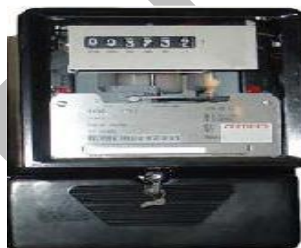
Figure 1: Traditional Energy Meter
