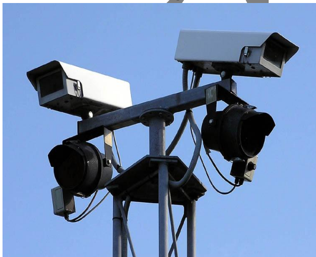
Fig. No. 2: Traffic signals with CCTV cameras
