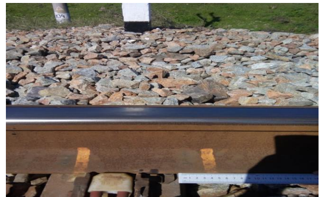
Figure 3. Marking of the control section on the lash and the "beacon" sleeper to control the hijacking of the track for the rail fasteners.
