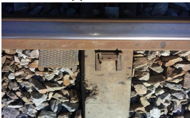
Figure 2. Displacement of the under-rail linings along the sleepers.
