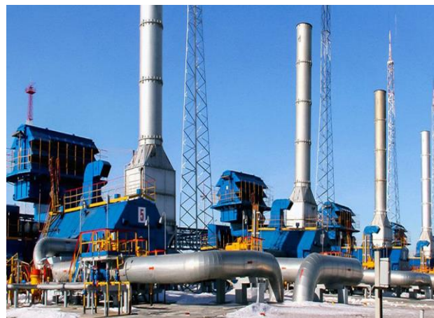
Fig. 2. Compressor station on a gas pipeline
