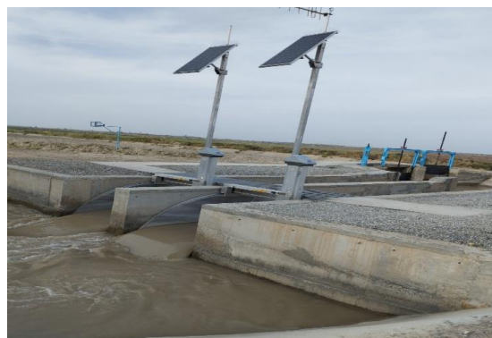
Figure 2. General view of the automation system of water objects "Rubicon Water" installed in the Qamashi-Mirishkor canal
