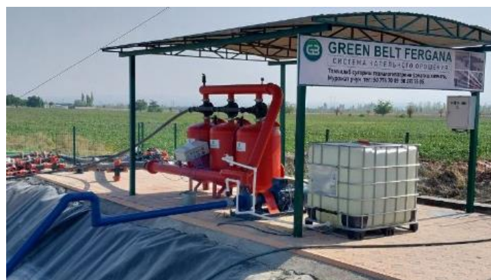
Figure 3. Overview of the automation system of water bodies used for irrigation of agricultural fields [7]
